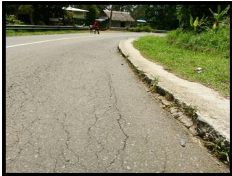
Figure 2. Ground cracks on the Palopo-North Toraja axis route
