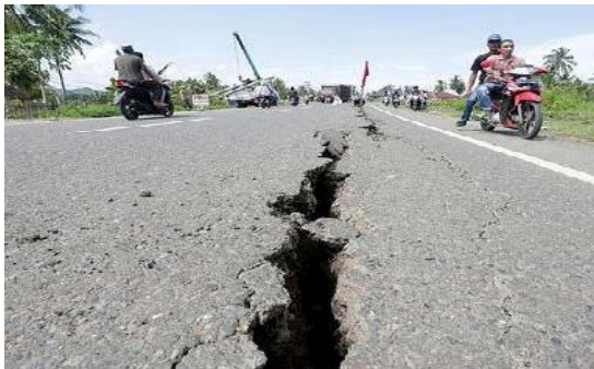
Fig 2. Rupture of an earthquake that occurred on December 7, 2016 in Pidie Jaya region, Aceh.
