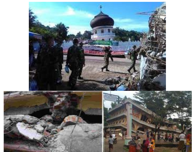
Fig.5. Repeat Failure that was detected in Pidie Jaya Earthquake victims December 7, 2016. (Source : https://bnpb.go.id/ ).
